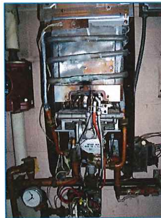
One of Six Obsolete Boilers
