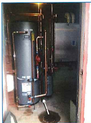
Central Boiler & Water Heater
