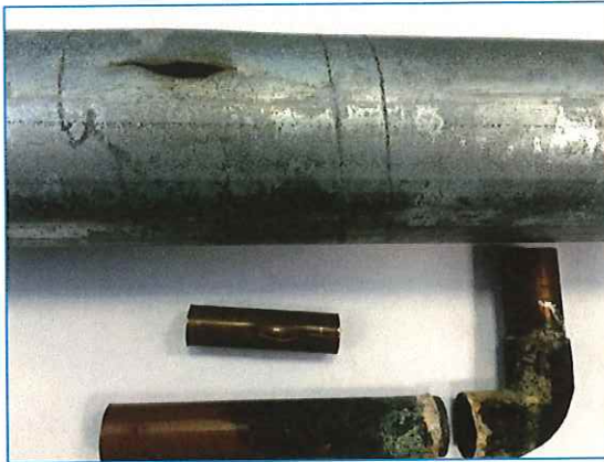
Frozen Pipe Damage & Defective Weld
