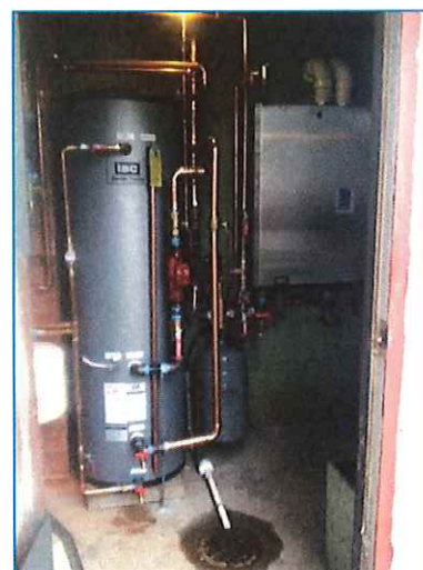
Enfield Manor Boiler & Water Heater
