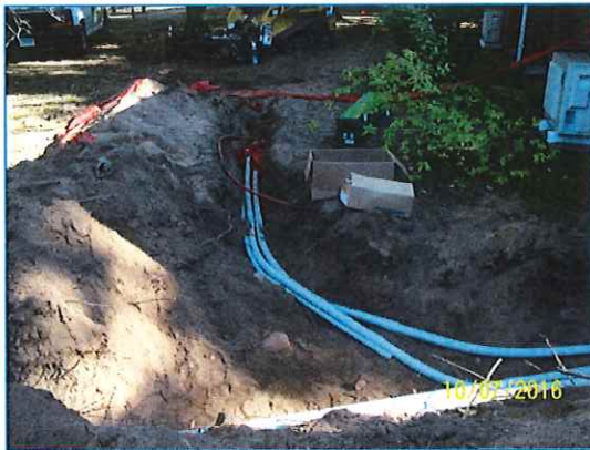
Electrical Cabling at Woodside Park
