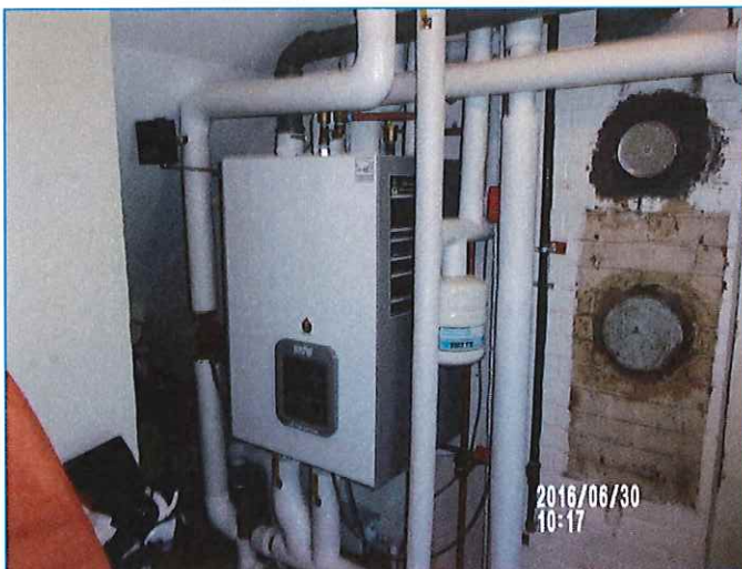
New Laurel Park Boiler
