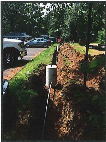
Site Lighting Bases & Wiring
